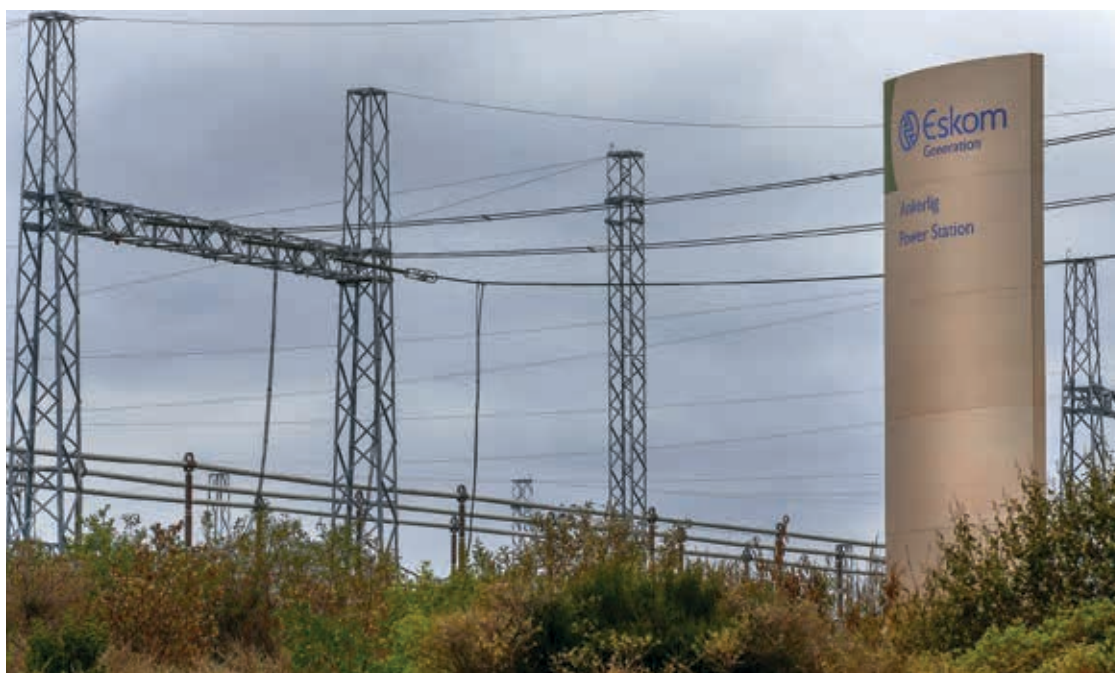
Eskom power station.
